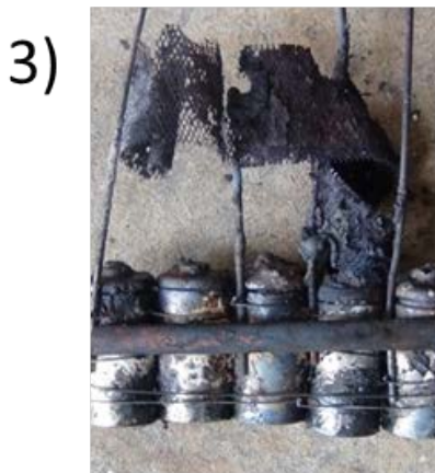
Internal components were partially ejected.
