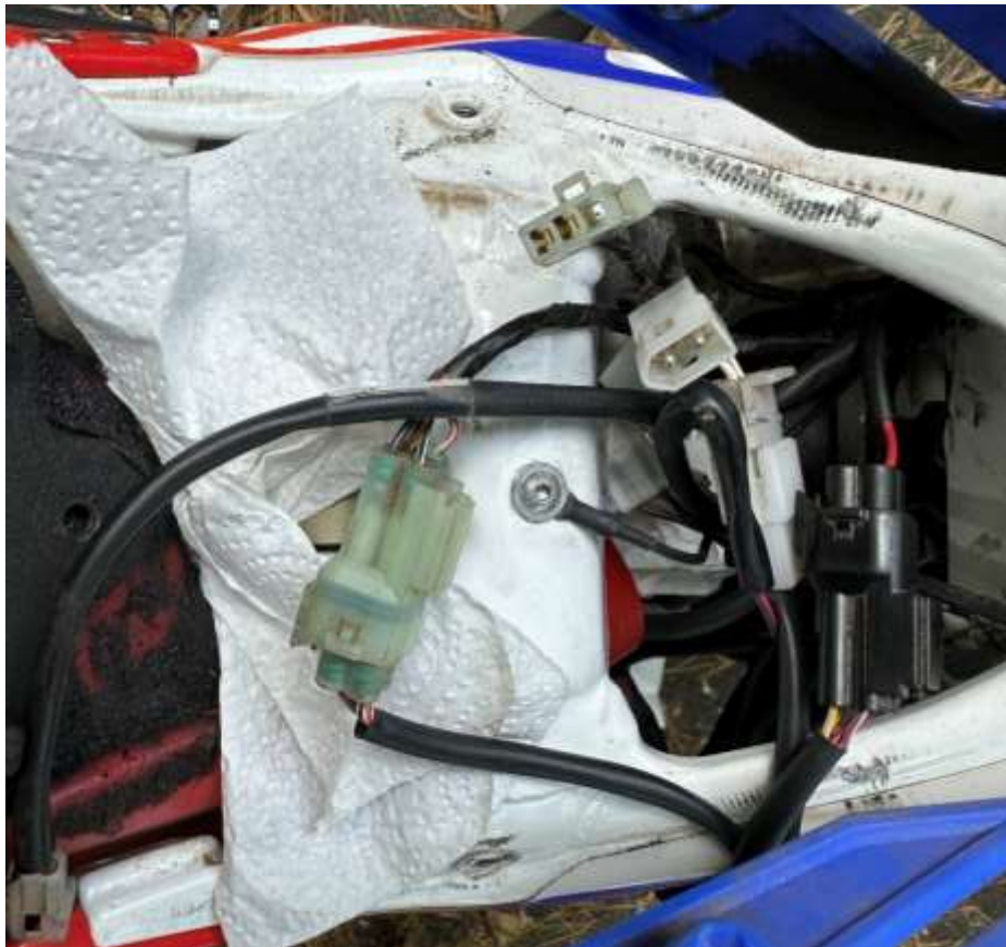
Figure 10 This is the return path for the spark plug current. It may not be adequate.
